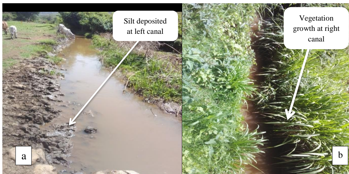
Figure 17 Silt deposited and vegetation growth at the main canal
