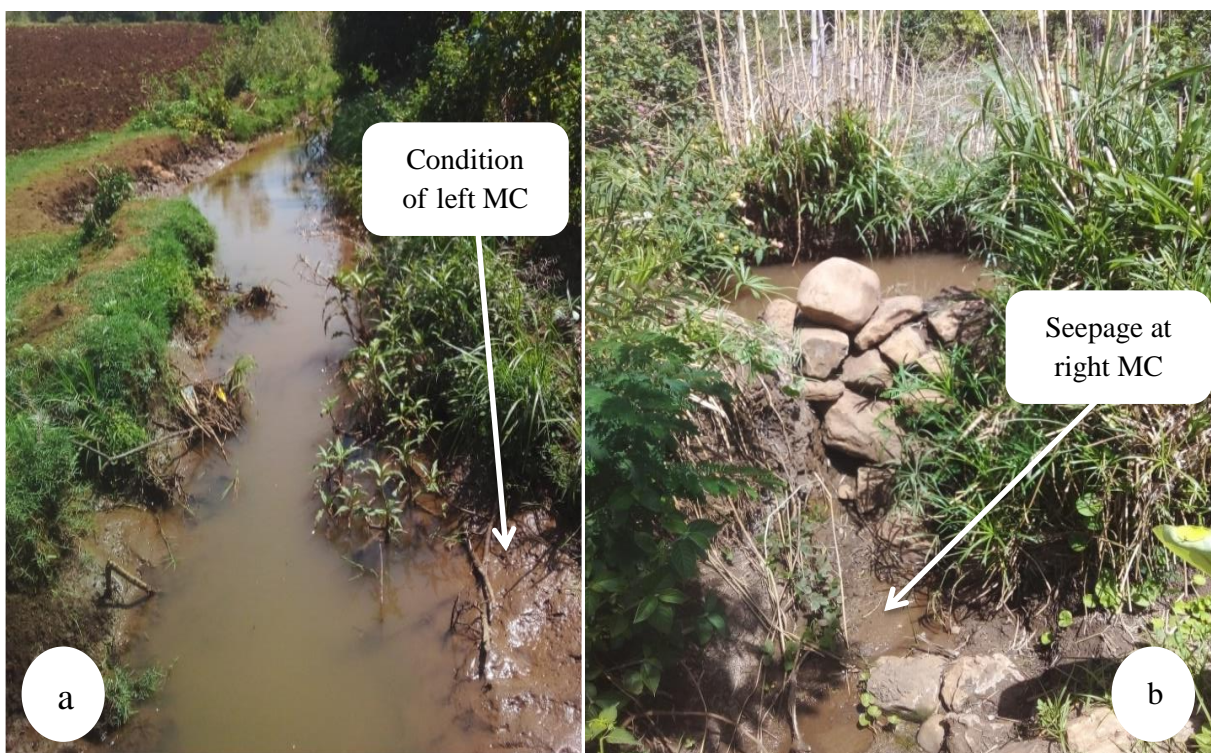
Appendix Figure 4 Canal condition and seepage loss
